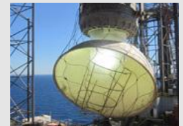
Light shade and impact guard dislodged due to corrosion
