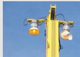
Crane boom light after collision
